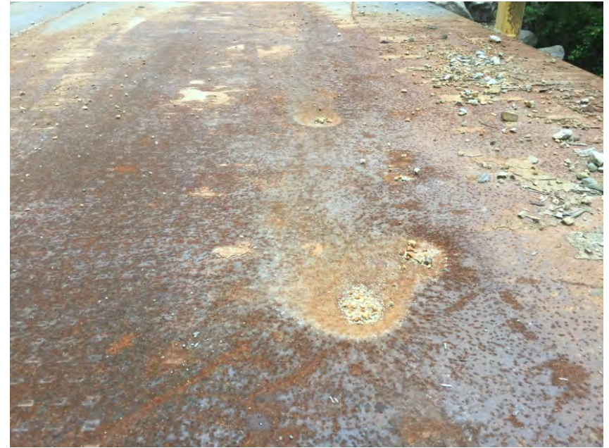
Minor deck deformation
